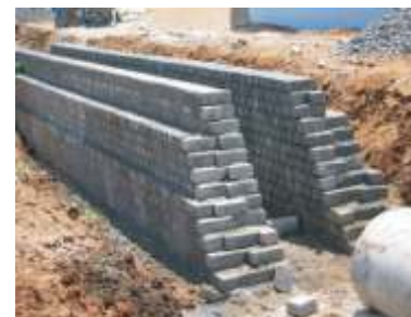
High strength FaL-G (20 MPa) blocks used in replacing concrete for construction of a culvert at the entrance of a market yard with traffic of over 2000 trucks a day (Vijayawada-A.P., India)
