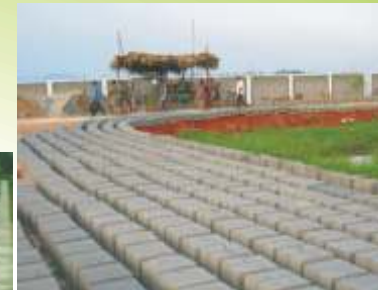
Production of FaL-G bricks as Road side activity in a massive housing colony under construction
