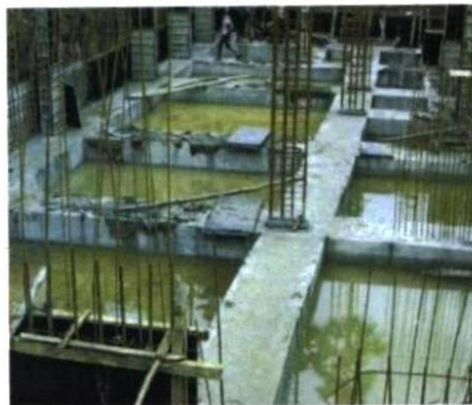
Raft Foundation with Dynamic concrete (170 kg of OPC/cu.m and strength of 40 MPa)
