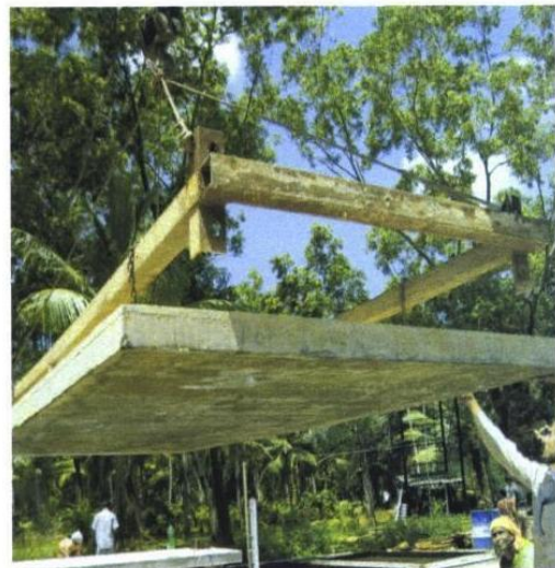
Precast roofing panel [5 x 2 mtr] with 50 MPa strength lifted on 7 th day
